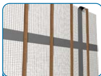
Tape overlapping joints with foil tape and fix 20mm battens to the Thermal Foil Bubble
